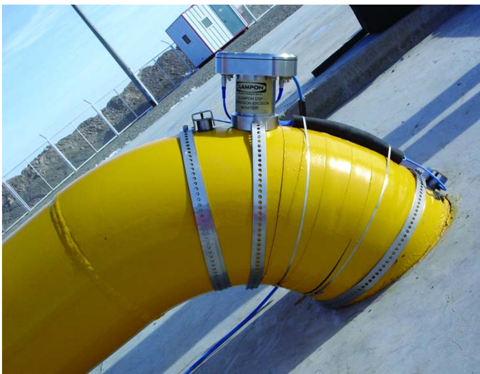
ClampOn CEM field installation.
